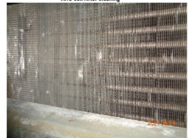
AHU Coil After Cleaning
