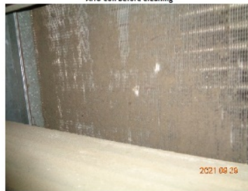
AHU Coil Before Cleaning
