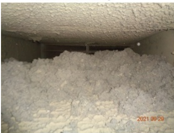
Lined Ductwork Before Cleaning
